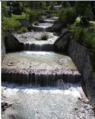
Series of consolidation weirs
